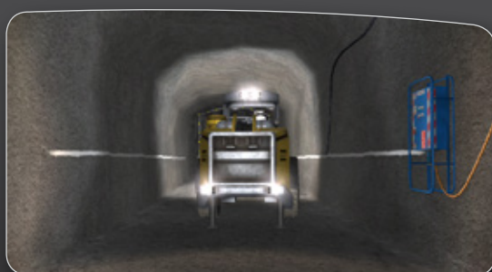
Connecting to Site Services
